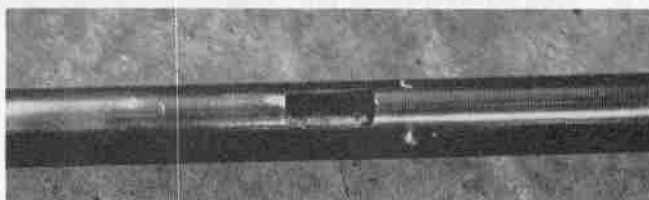
Holes are welded, fusing bushing to receiver body. If welds are built up above the surface and dressed back flush, no evidence of welding will be seen.
